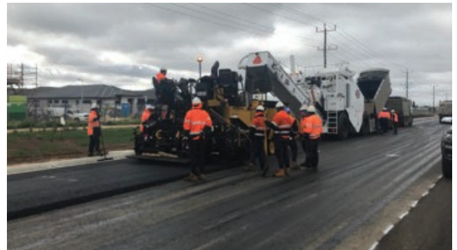
Figure 5: Western Roads Upgrade using recycled materials such as reclaimed asphalt pavement (RAP), crushed concrete and crushed glass
